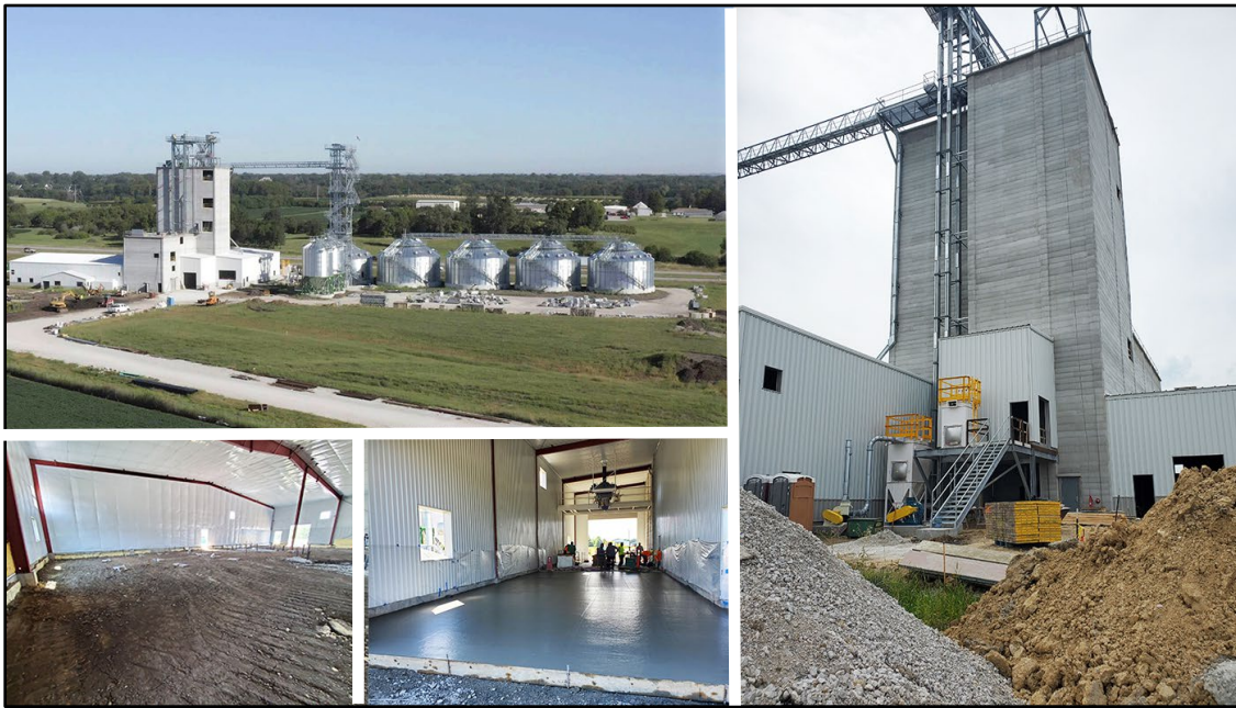
Iowa State University Kent Corporation Feed Mill and Grain Science Complex, recent progress
